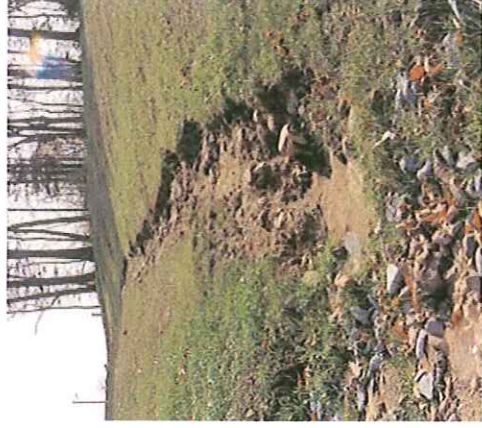
Remedial maintenance is necessary when some part of the facility deteriorates due to aging or damage, such as the excessive erosion in this snail.
