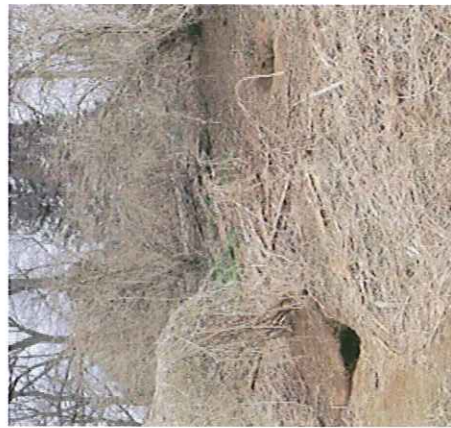
Constructed stormwater basin berms can be damaged by burrowing animals. This can lead to possible failure of the basin.
